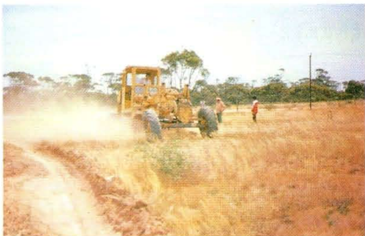
66. KOONIBBA, SA, AUSTRALIA. A swale under construction using a side-casting grader in the drylands of central southern Australia.
